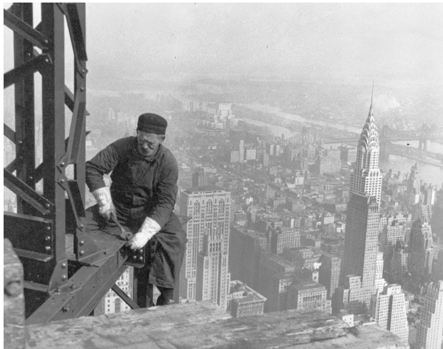
Figure 1-12 The Empire State Building was built in the record time (for its era) of 20 months. The contractors accomplished this through the creation of new procedures and details of construction designed specifically for the type of project and the schedule. Lewis Wickes Hine, National Archives.
