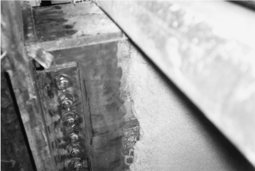
Figure 1.15 Left: crack in beam web during the Northridge earthquake, Anthony Building, Department of Water and Power, Los Angeles County.
