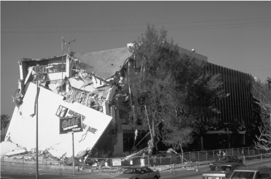
Figure 1.7 Northridge earthquake, 1994. Collapsed end shear wall, Kaiser Permanente Office Building, Granada Hills, CA. (Photo courtesy of the University of California Library at Berkeley.)
