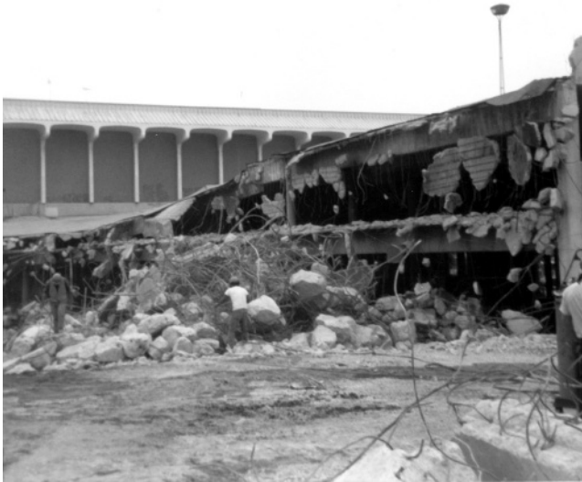
Figure 1.20 Collapsed upper floor and a large portion of the collapsed parking structure, later demolished, Whittier Narrows earthquake, 1987.
