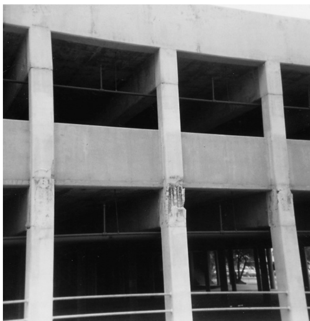
Figure 1.18 Initial stages of column joint degradation in the progressive failure of a fashion center parking structure in the Whittier Narrows earthquake, 1987.
