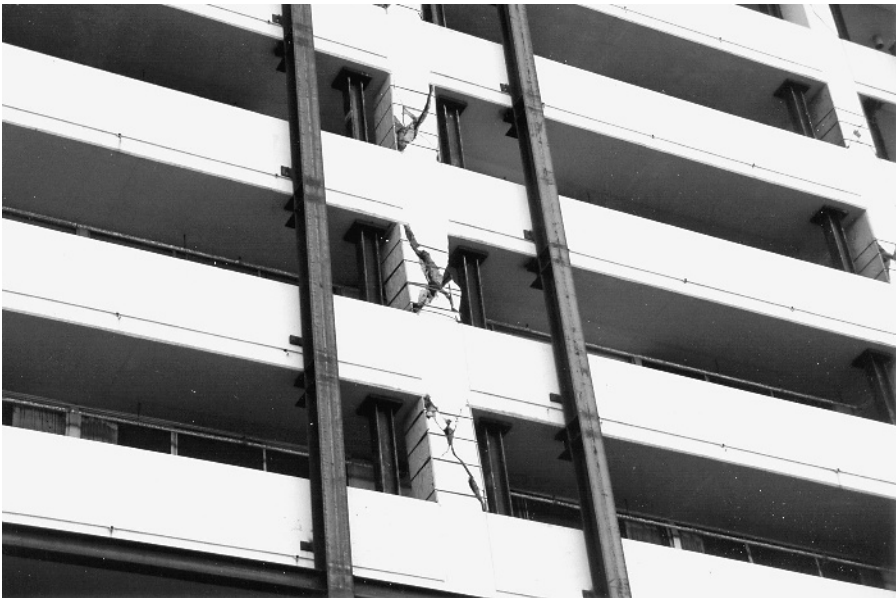
Figure 1.9 Reinforced-concrete columns severely damaged in the Northridge earthquake, Champagne Towers, Santa Monica, CA.
