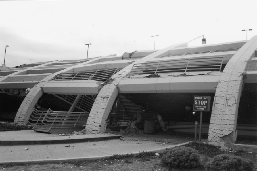
Figure 1.1 Parking structure that collapsed during the 1994 Northridge earthquake, California State University, Northridge Campus.
