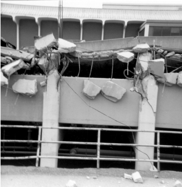
Figure 1.19 Exterior columns that supported the second floor broke at the second-floor beam–column intersection, fashion center parking structure.
