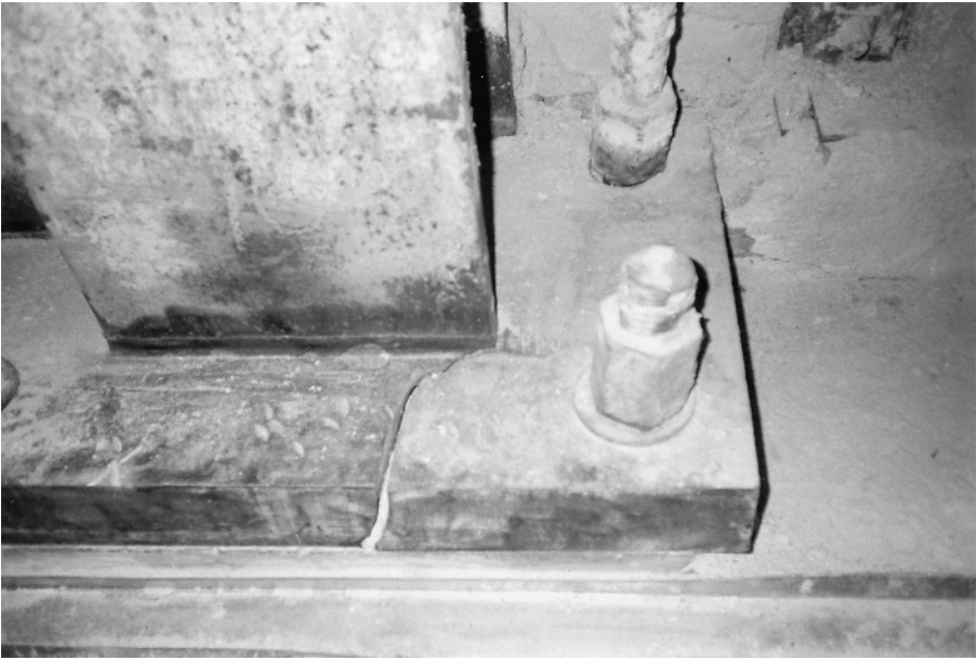
Figure 1.16 Cracks in 4-in.-thick base plates during the Northridge earthquake, Oviatt Library Annex Building.
