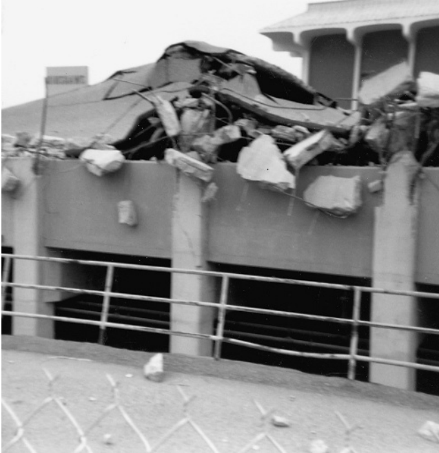
Figure 1.3 Detail of parking structure that collapsed during the Whittier Narrows earthquake of 1987.
