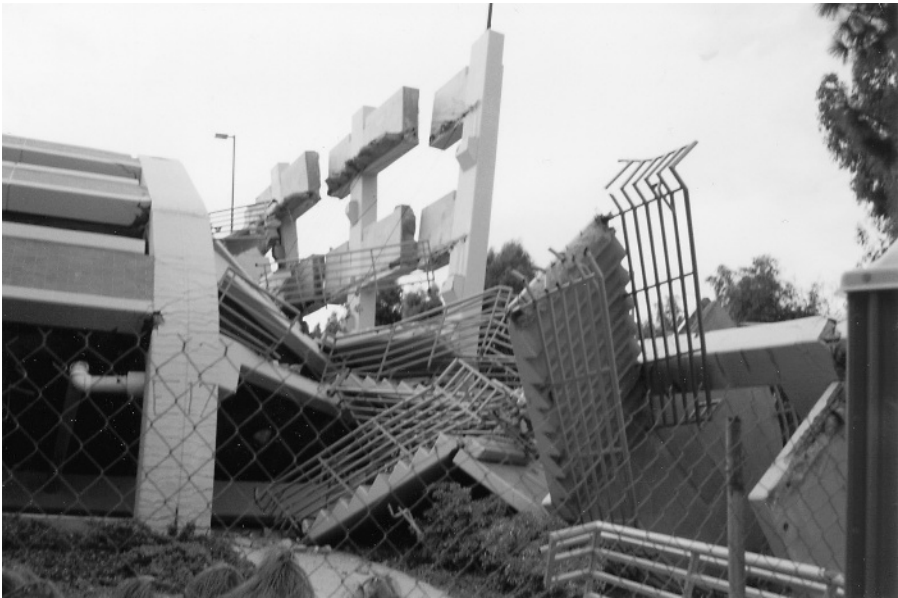
Figure 1.14 California State University parking structure. A corner of the cast-in-place framework was pulled in by the collapsed interior of the multistory structure during the 1994 Northridge earthquake.
