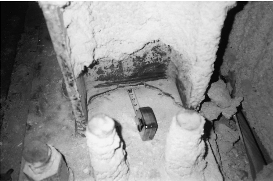
Figure 1.17 Shear failure at perimeter of frame leg–base plate solidly welded connection, Oviatt Library Annex Building. Note the crack in the center and the initial stage of shear failure on the left.
